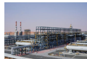
Abu Dhabi Onshore Concession Oil processing facility
