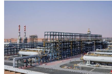
Abu Dhabi Onshore Concession Oil processing facility
