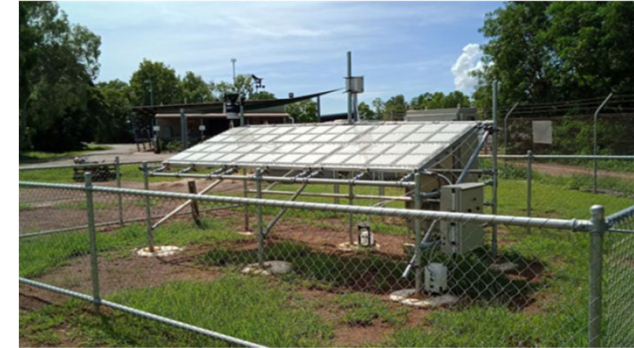
Artificial photosynthesis panels installed in Darwin, Australia
