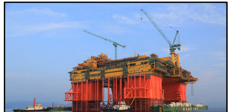
Launched central processing facility (September/2015)
