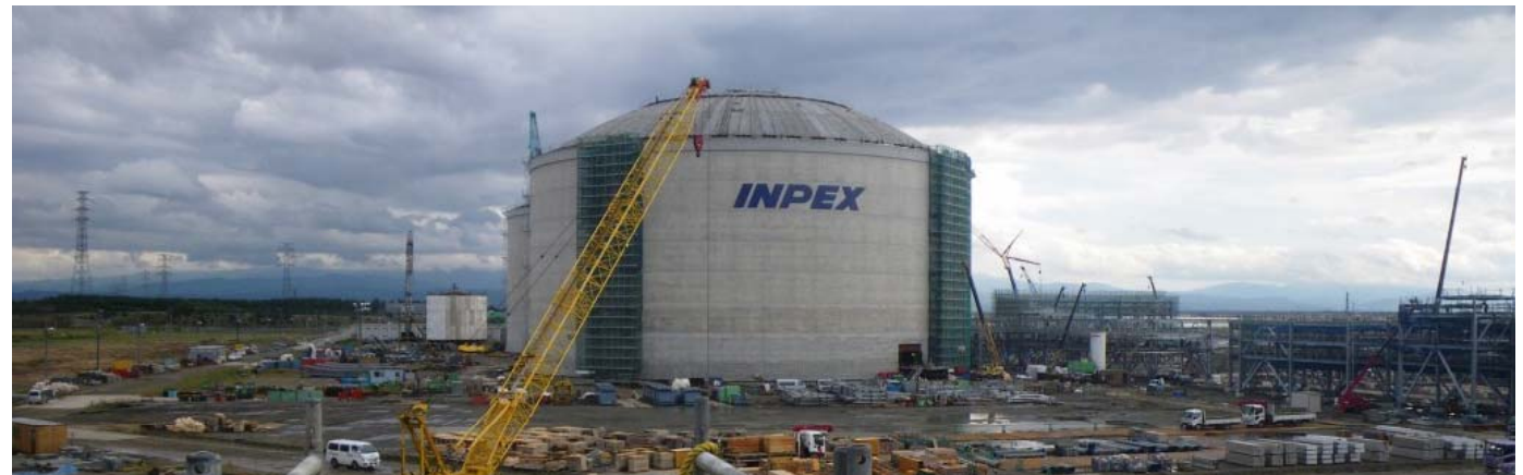
(LNG tanks, as of October 2011)
