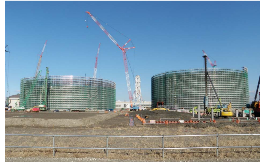
(LNG storage tanks, as of January 2011)
