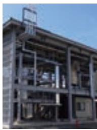
Demonstration facility at the Koshijihara Plant
