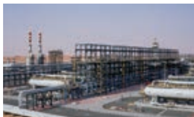
Abu Dhabi Onshore Concession (oil processing facility)
