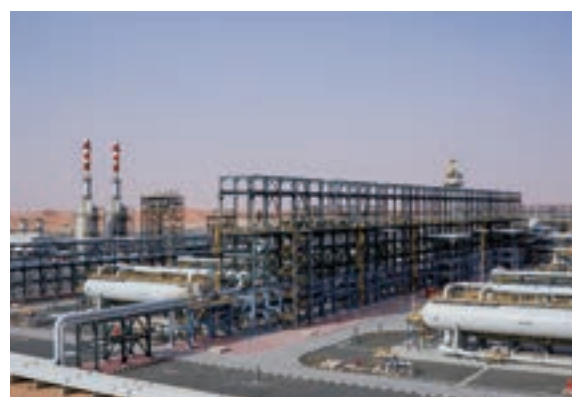
Oil processing facility
