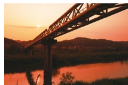
Natural gas pipeline that crosses a river (Shibumi River, Niigata Prefecture)
