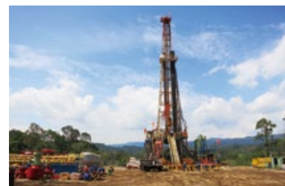
Sarulla Geothermal Independent Power Producer (IPP) Project
