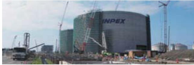
Construction at the Naoetsu LNG Receiving Terminal
