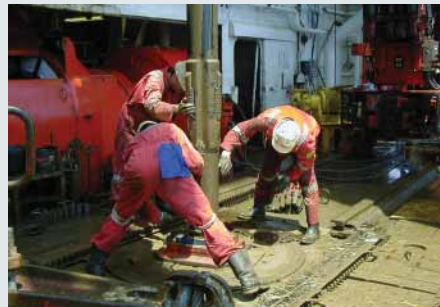
Operation in Offshore Western Australia
