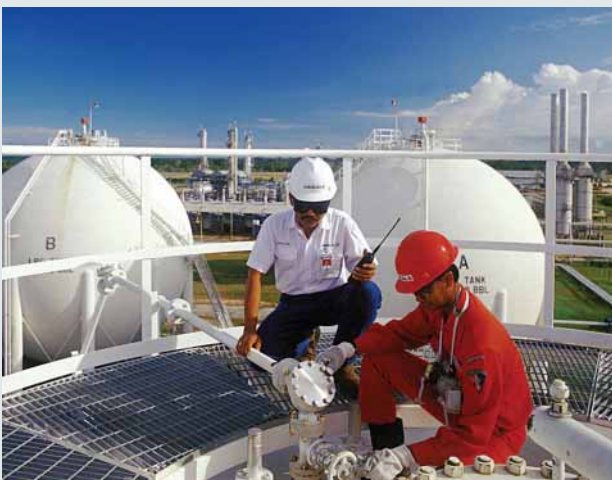
Santan LPG Storage Facility
